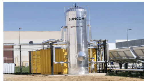
Figure 2: an operational TES built by Suncom for a project in Spain
